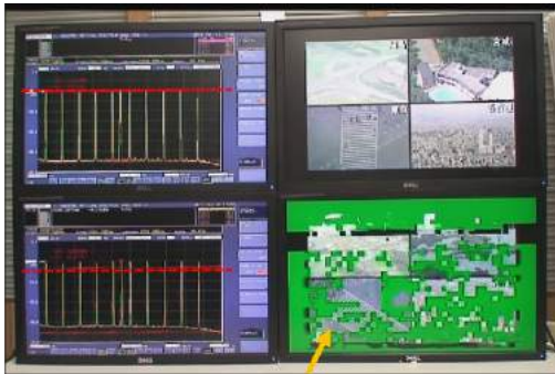
Receiving error due to high-power optical path (b) 10 wavelengths (top) service continues (bottom) service is disrupted.
